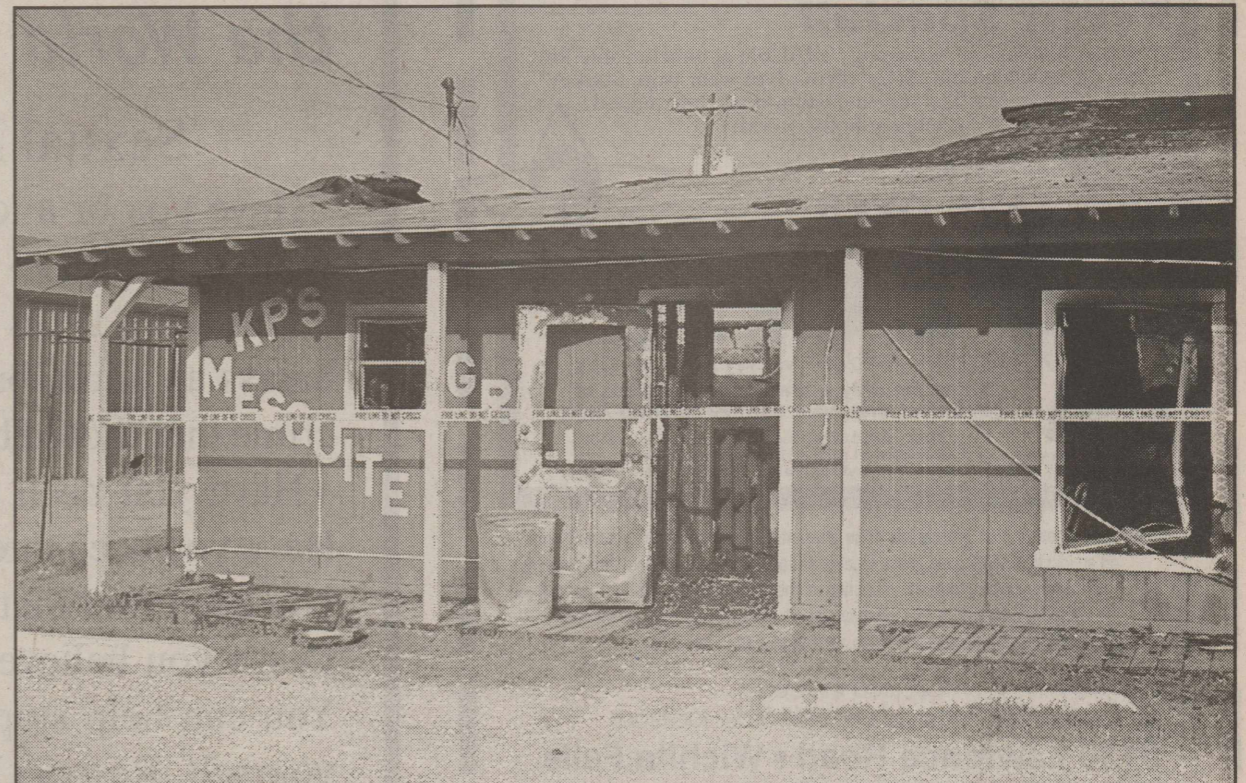
KP'S RESTAURANT DESTROYED —At about 2:40 Friday morning, Haskell Volunteer Fire Department members responded to a fire that destroyed KP's Mesquite Grill, located at 900 S. Ave. E. The fire was out about 3:45 a.m., but firemen stayed at the scene until about 5:00 a.m. trying to determine the cause. Haskell Fire Chief Bill Steele reported Monday morning that the cause was still undetermined.
