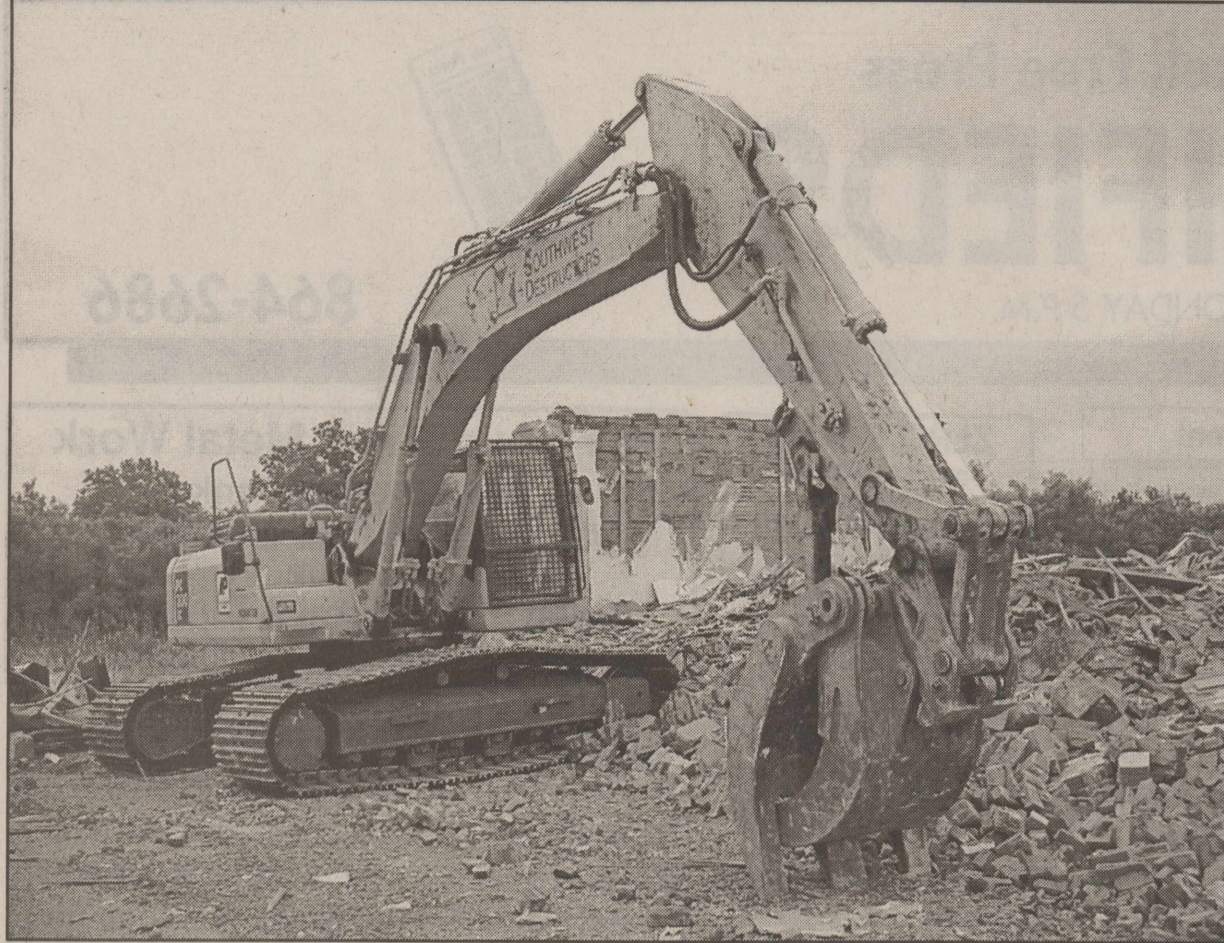
AND THE WALLS CAME TUMBLING DOWN—Demolition of the old Haskell ice house was part of the work done this week in making way for the new highway construction through the city.
