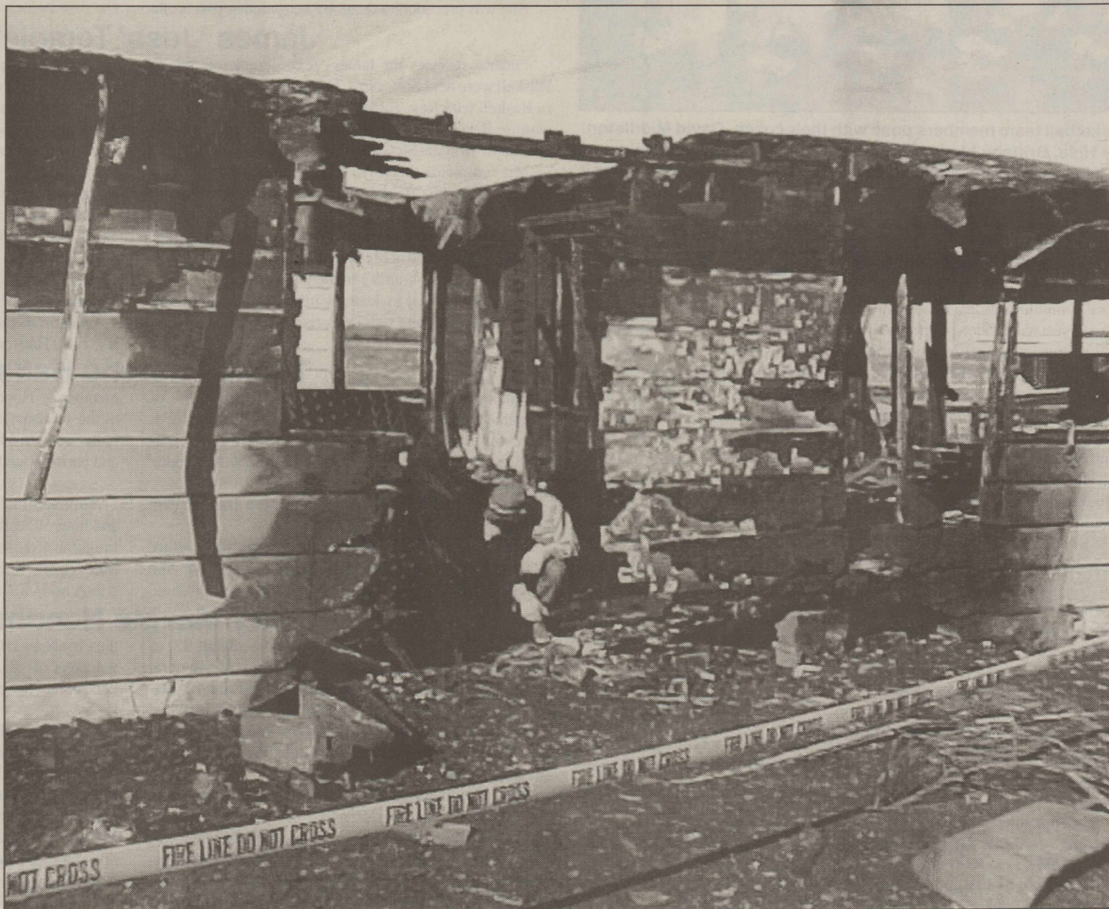
EARLY MORNING HOUSE FIRE -Haskell Volunteer Firemen responded to a call at approximately 4:15 a.m. Mon., Dec. 2, to a
