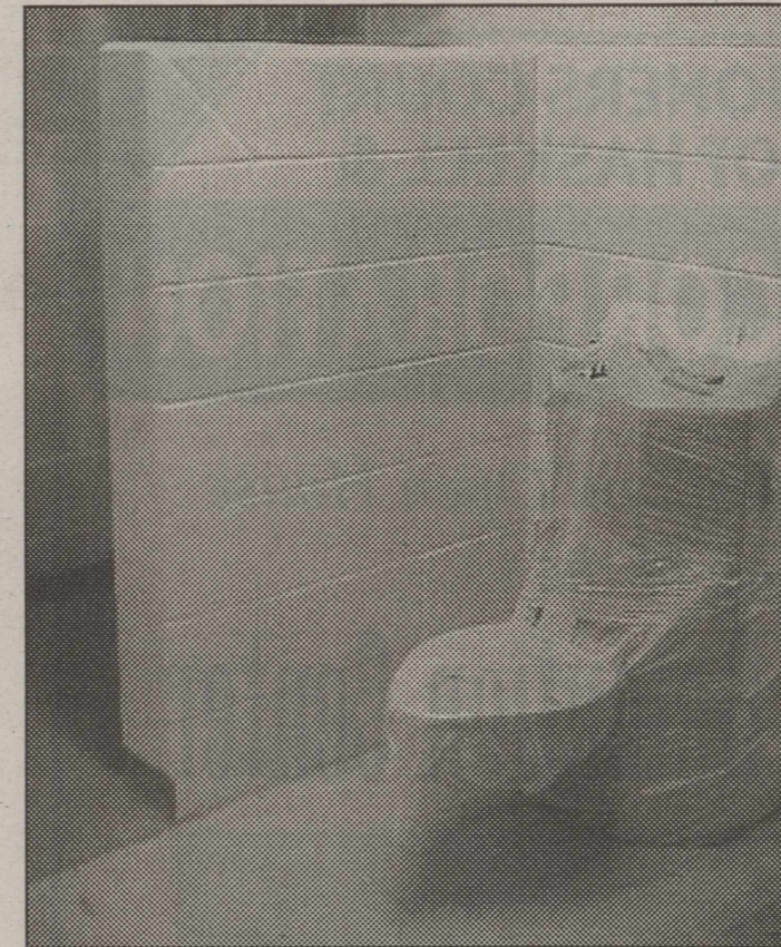
JAIL ACCOMMODATIONS—Bath facilities installed in cells at the Rolling Plains Regional Jail include only a single-unit stainless steel commode and lavatory and an open shower stall.
