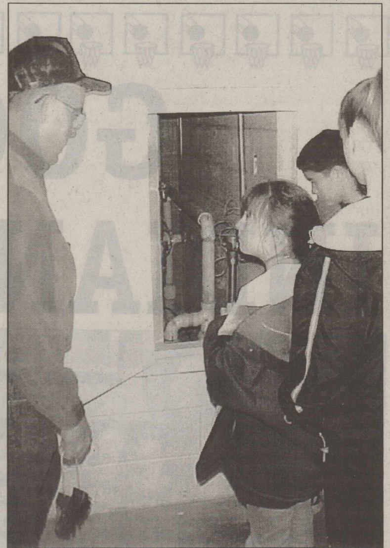
LOOKING AT THE PLUMBING—Holding the keys as they tour the Regional Jail, Billy Wayne Hester shows Haskell students one of the plumbing chase access areas located in the facility.
