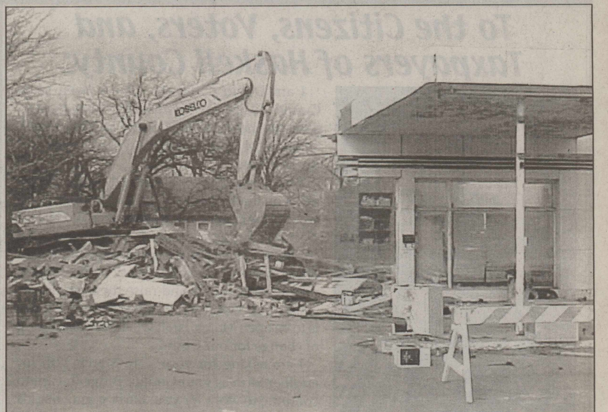
GONE IN A FEW GULPS—The old Gulf station that stood for years on the corner just north of the square in Haskell was demolished and hauled away this week. Underground gas tanks were removed and the buildings leveled by work crews in only two days, clearing the way for progress by the City.
