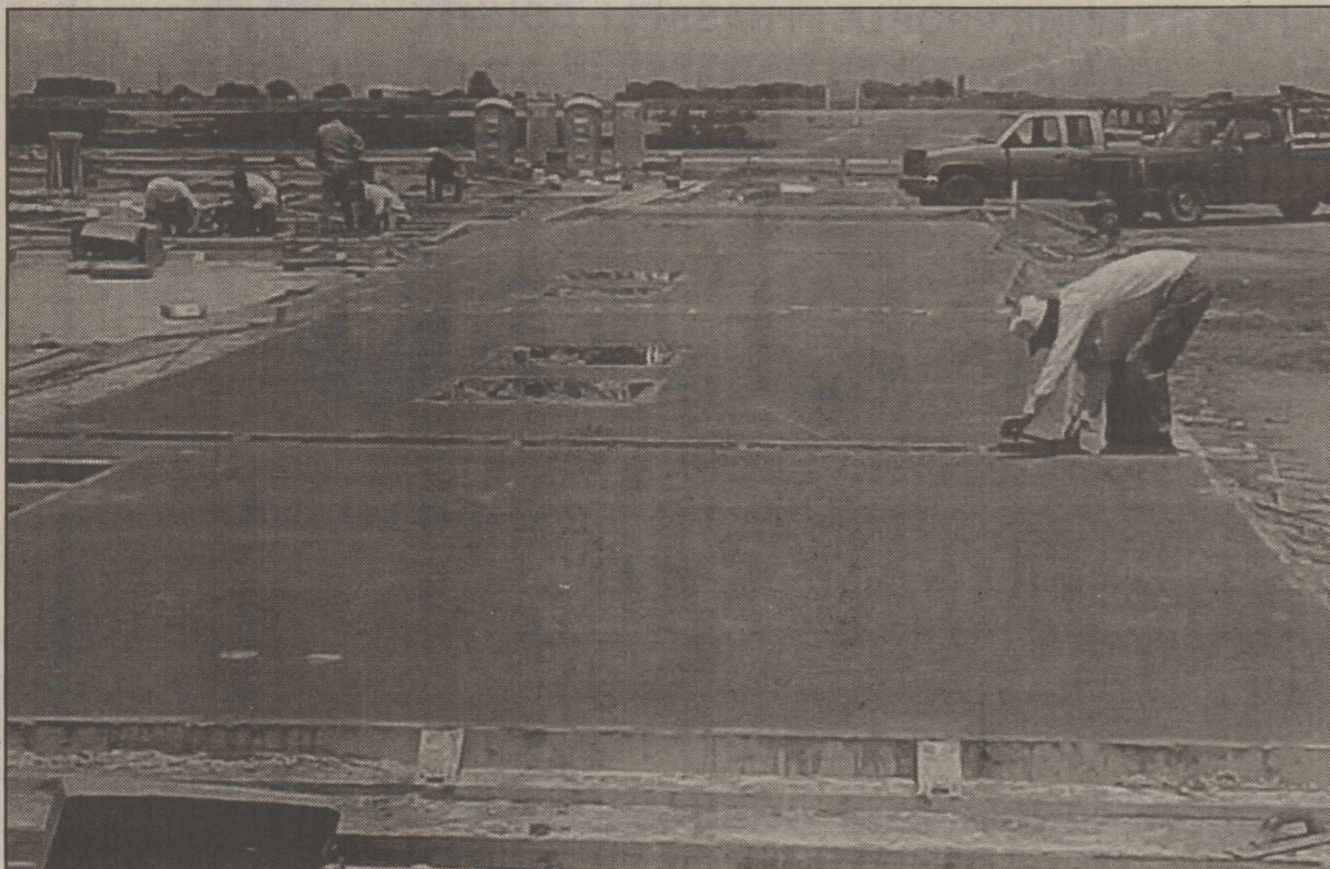
POURING WALLS—Crews work to pour cement into forms on the ground where they will be cured before being lifted into place by crane, forming the exterior walls at the Regional Detention Center.
