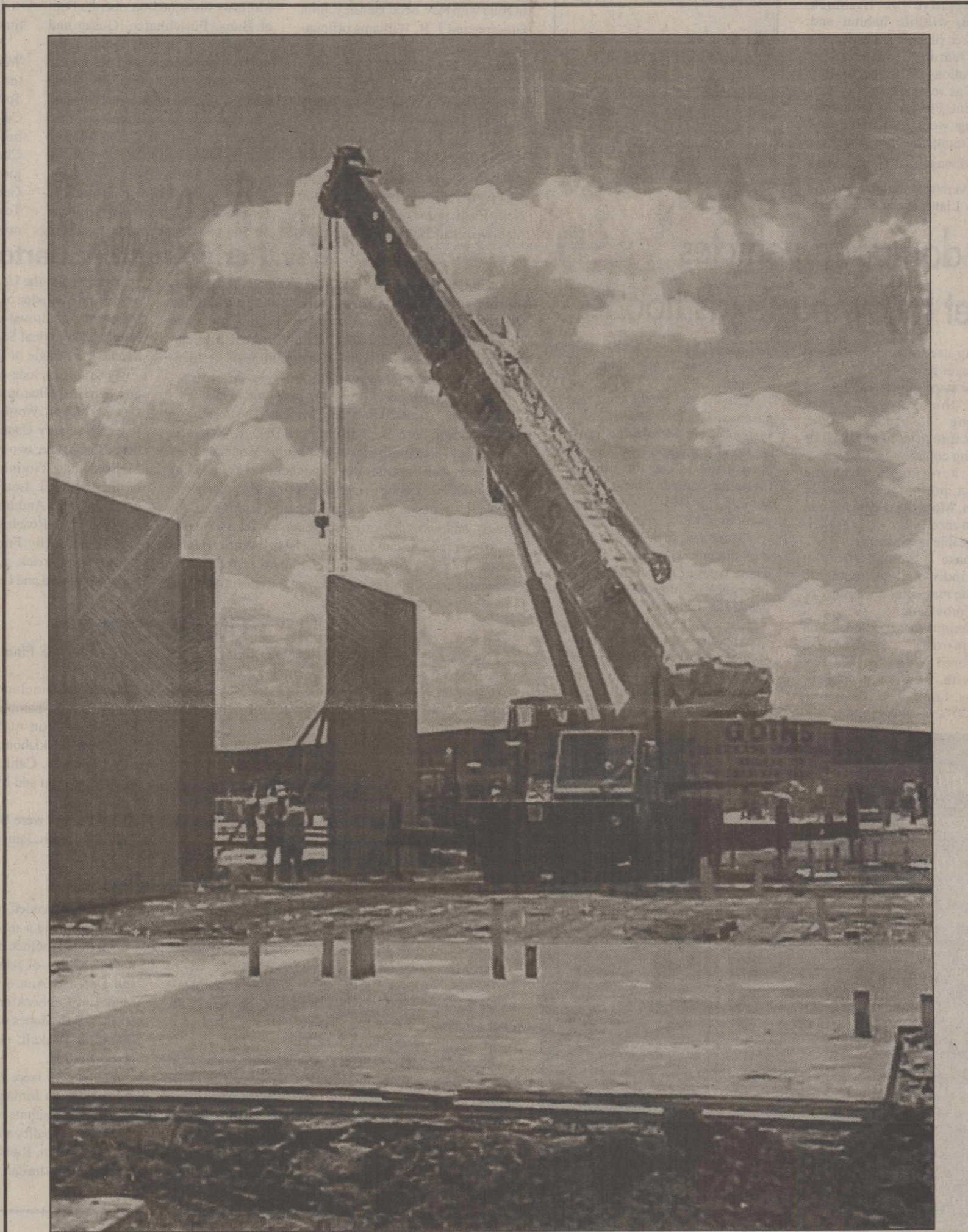
RAISING PRISON WALLS—The heavy construction crane lifts and sets sections of concrete exterior walls in place at the Regional Detention Center construction site in Haskell.
