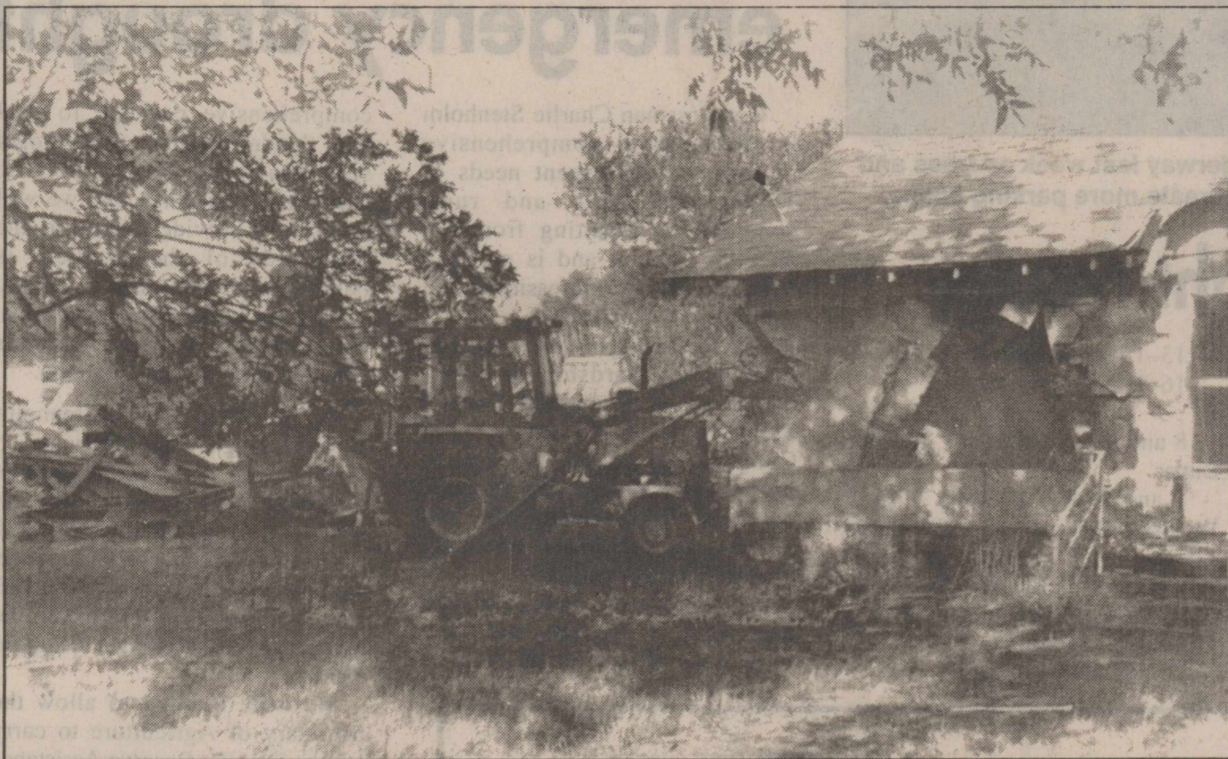
DEMOLITION —Making room for the new expansion of Burkett's Family Restaurant, outbuildings and a house were demolished last week on two lots north of the business on Hwy. 277.
