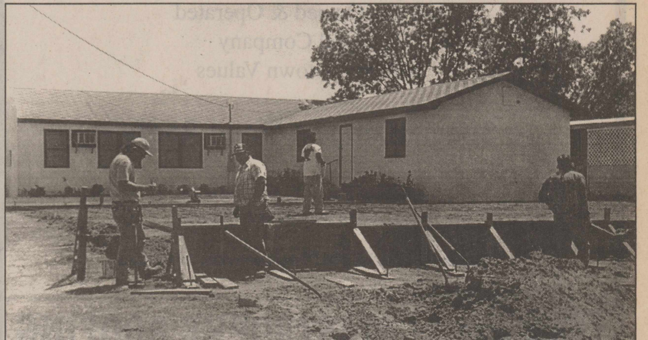
NEW ADDITION —Work began this week on a new sanctuary for New Covenant Foursquare Church of Haskell. The present sanctuary will be used for a fellowship hall later. On completion, of the outside building, members of the church plan to do all of the inside finish work themselves.
