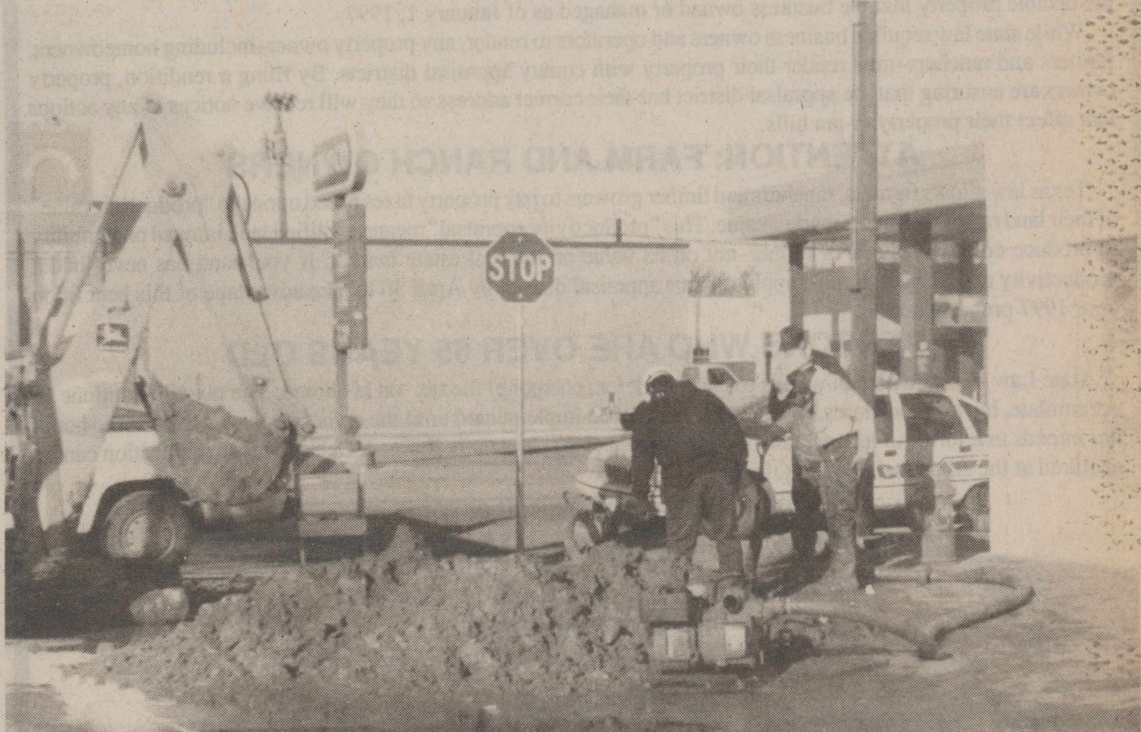
WATER LEAK —City employees are shown working on a water leak at the corner of North 2nd Street and Hwy. 277. Several water leaks occurred during the week as freezing temperatures gave way to warmer weather conditions. Parts of the city were without water for a brief period while employees worked to repair the leaks.
