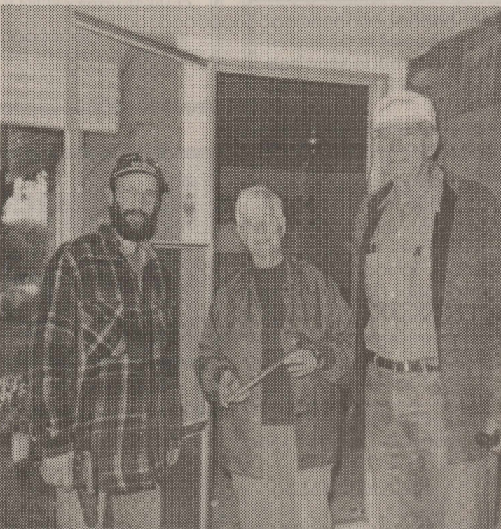
INSTALLING A STORM DOOR—Allen Barnett (from left), Frankie Smith and Bob McCowen.
