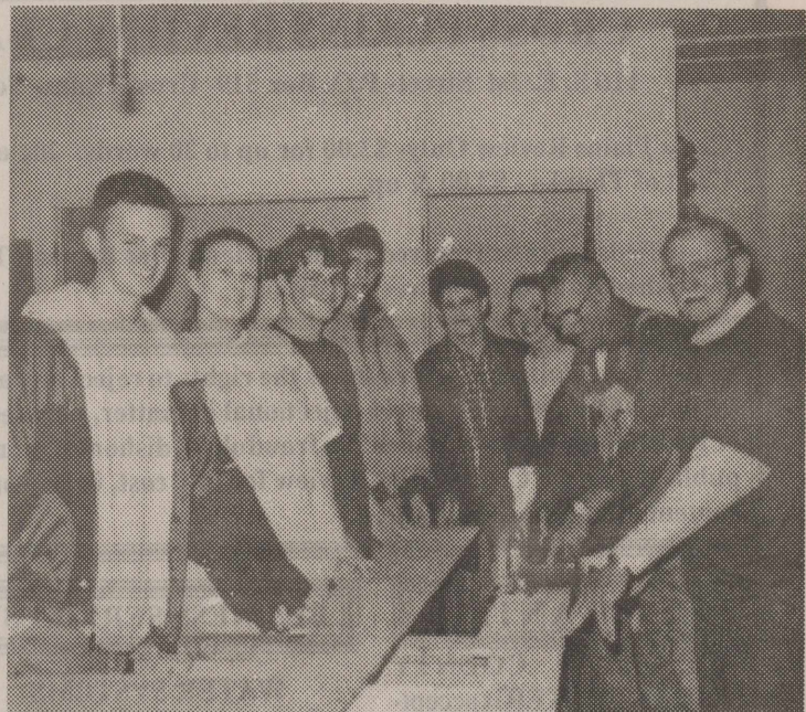
REPAIRING A WHEEL CHAIR RAMP—Walter Thomason and Bob Pipes (far right) and members of the Key Club and Honor Society.
