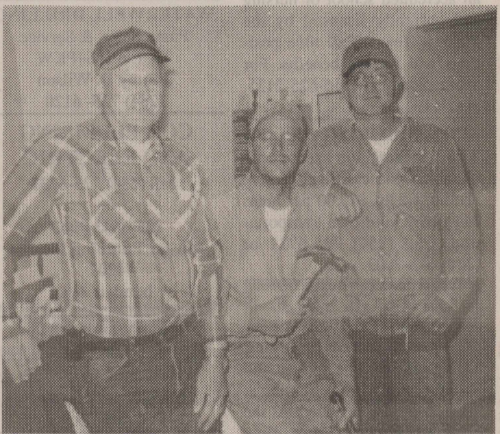
WORKING ON CEILING REPAIRS—John Swift (from left), Bryan Bennett and Wes Castleman.
