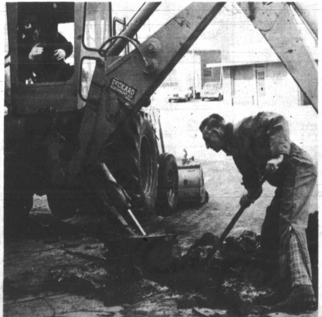
CITY EMPLOYEES repair a broken water line along the 300 block of W. Foster Friday. (Pampa News photo by John Price)
