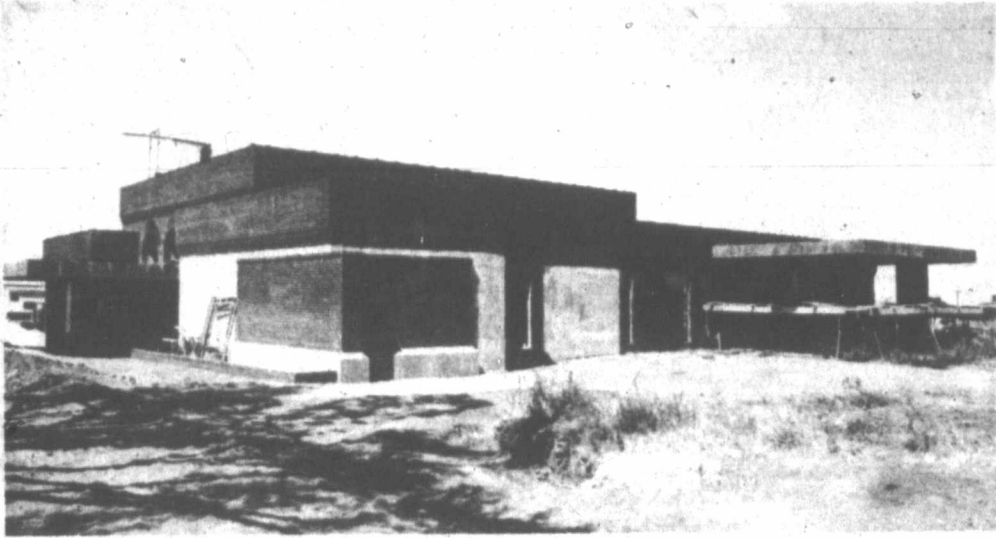
THE NEW First National Bank in Wheeler is nearing completion. The building is being built at the intersection of Alan L. Bean Boulevard (Highway 83) and Texas Road. High Plains Builders of Amarillo is the general contractor.
