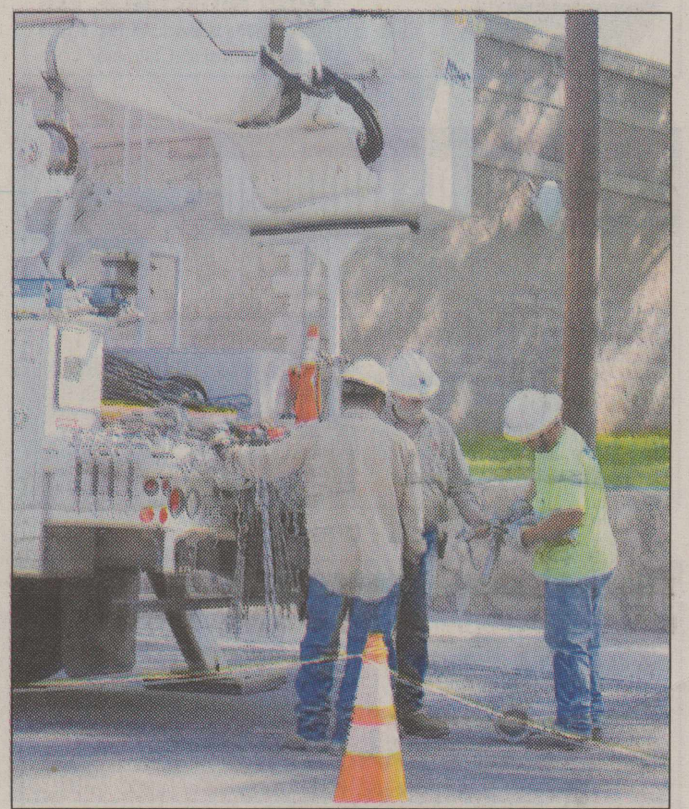
Foreman Richard Hall (center), of B&B Electrical & Utility Contractors, oversees work to replace a pole and upgrade electrical wires, Monday, July 17, 2017, along Water Street, near downtown Sonora.
