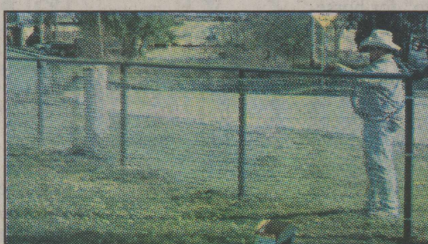
Rowdy Buell finishes work on the new fence surrounding the city softball field.
