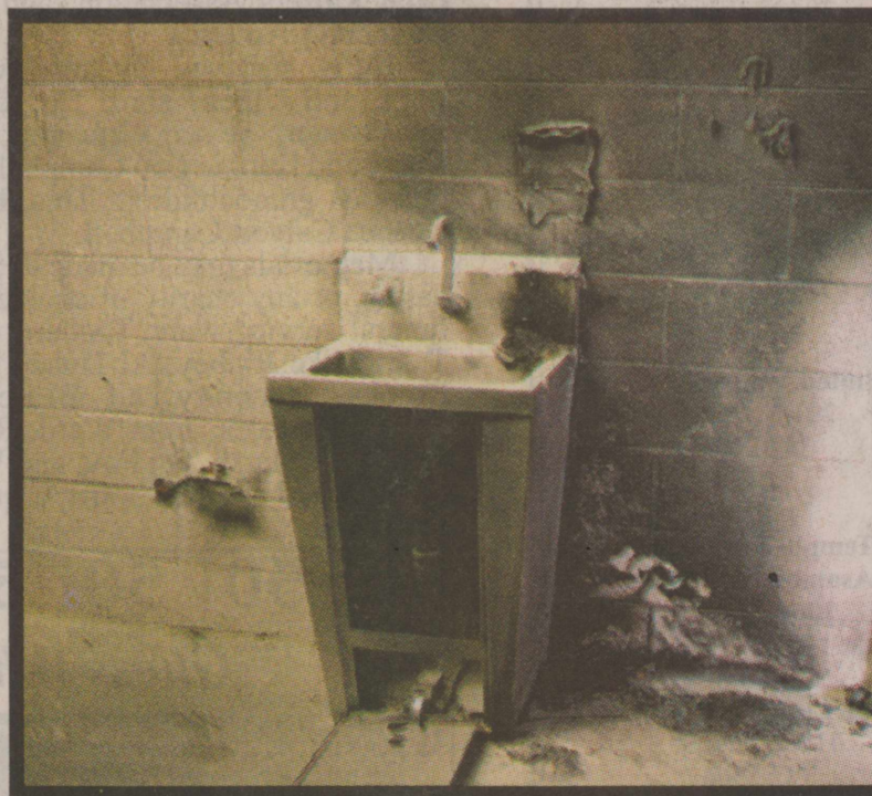
Smoke damage to the restrooms will cost up to $600.
