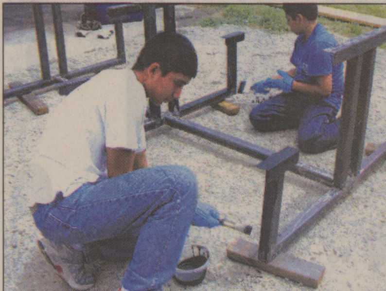
Sonora Sophomore, Paul Faz, completes construction on one of two picnic benches to be placed on Eaton Hill
