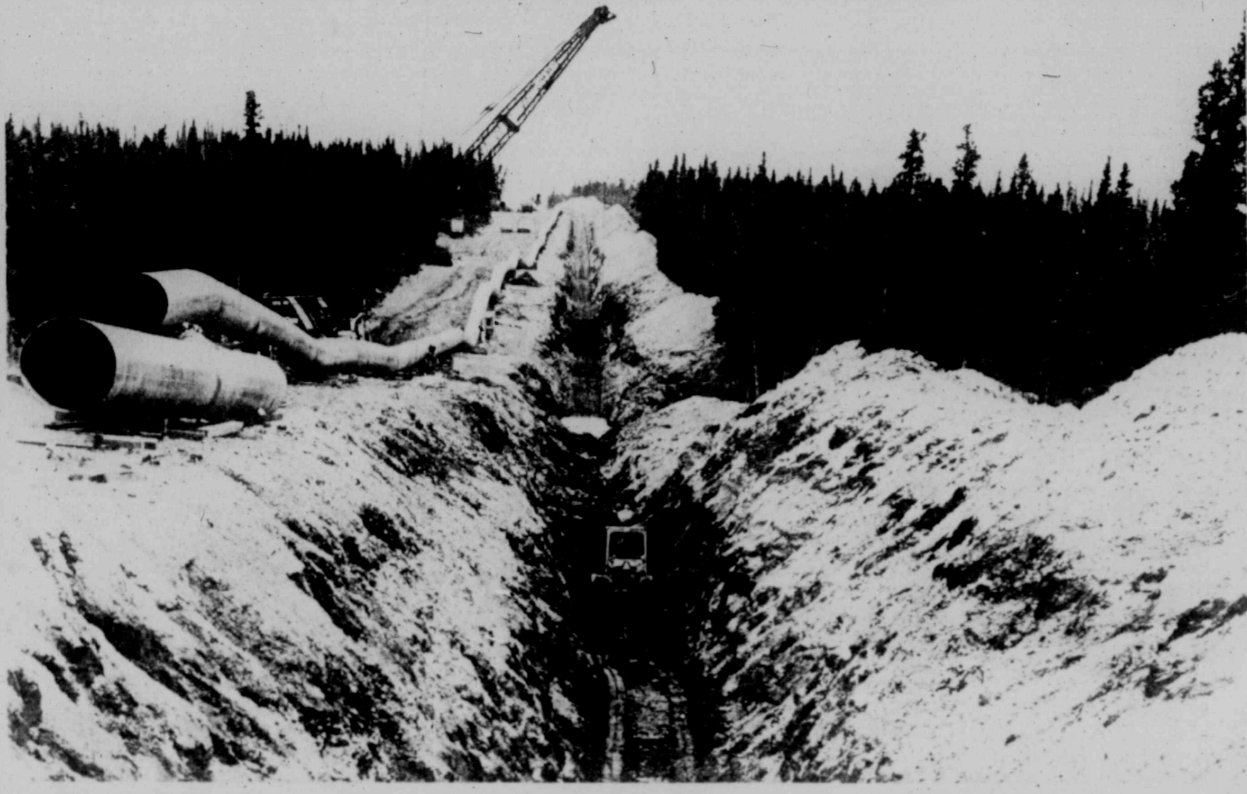
A TRENCH IS prepared for a section of the trans-Alaska pipeline about 225 miles north of Valdez. About 400 miles of the
