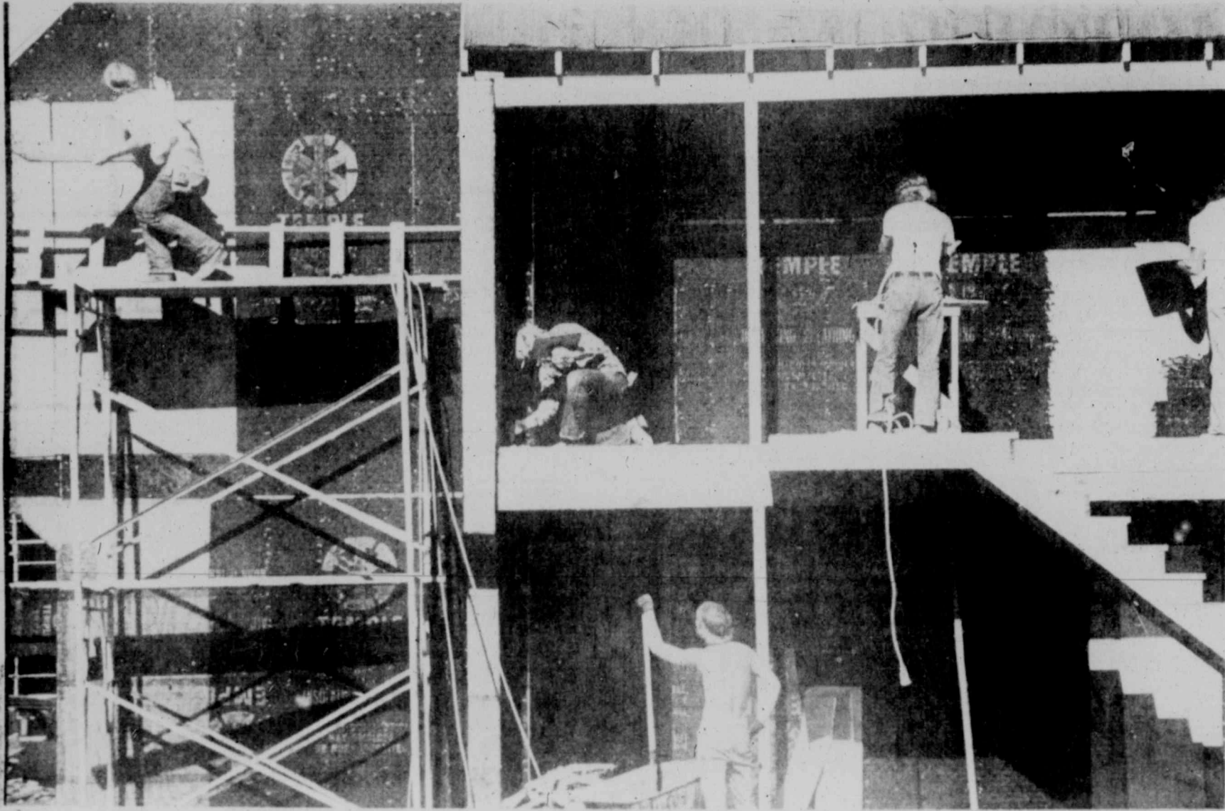
IF YOU LET your imagination run rampant you can vision that these workmen are preparing for a game of Hollywood Squares, but the more realistic viewer will see workmen hurrying to complete one of Midland's newest living complexes, the Haystack Apartments in the north part of Midland.
