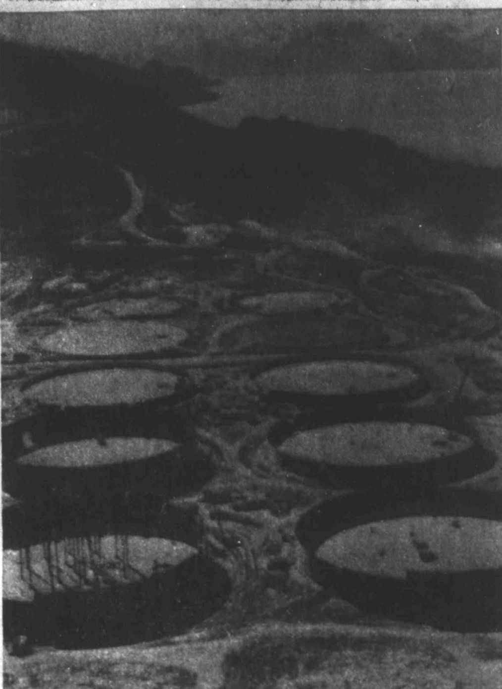
VALDEZ STORAGE TANKS - Crude oil storage tanks take shape at the Valdez, Alaska, terminal site for the trans-Alaska pipeline. Eighteen of the half-million barrel capacity tanks will be built to handle the pipelines initial 1.2 million barrels per day. Each tank will hold an internal steel structure, being erected in front left tank, to support a cone-shaped roof required for heavy winter accumulations of snow. (AP Wirephoto.)
