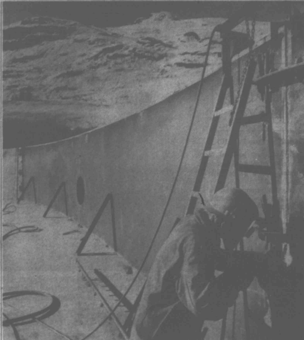
PREPARING FOR DELIVERY — A welder joins two segments of steel rings for a 250-foot diameter crude oil storage tank being constructed at the Valdez terminal of the trans-Alaska pipeline. The tank, which will be 62 feet high, will have a capacity of 510,000 barrels of oil. Eighteen tanks are being constructed to take the initial pipeline deliveries.
