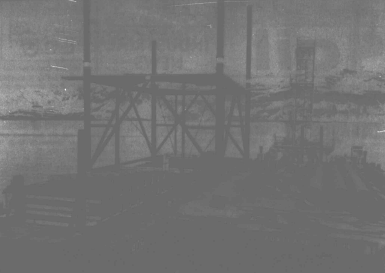
BERTHS AT VALDEZ — This equipment is being used on the trans Alaska pipeline project for drilling footings for the tanker berths at Valdez, the terminus of the 800-mile-long pipeline. Four tanker berths are being built in the first phase of construction.
