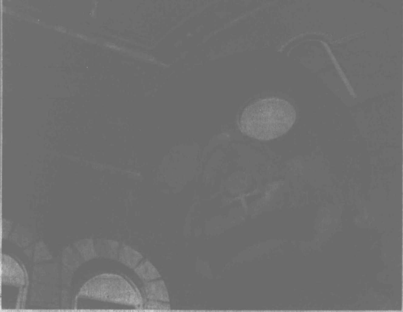
OPERATION FACELIFT—Workman Joe Mayer wears a mask to protect himself from brick dust during renovation of Holy Trinity Cathedral, a landmark in New Ulm, Minn. (AP Wirephoto.)
