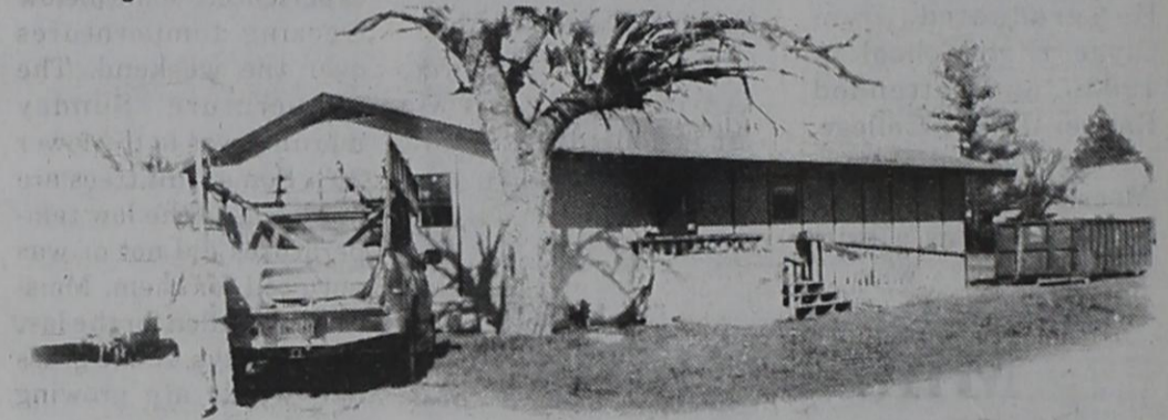
Top: New Baird motel goes up. Bottom: New Day Care Center being built.
