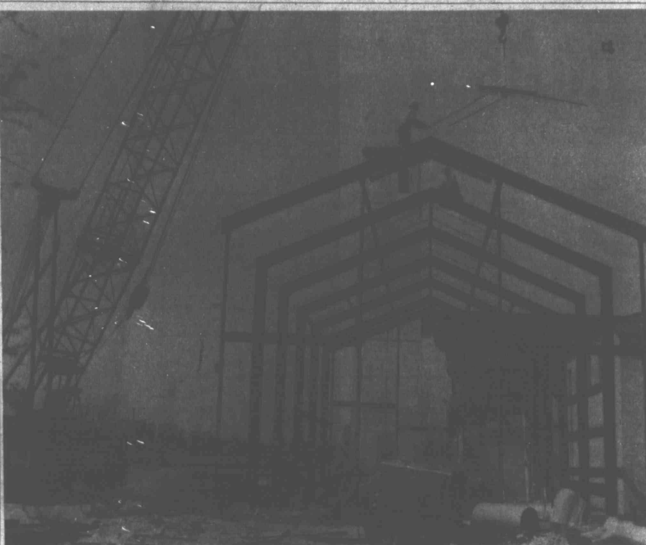
TOPPED OUT — Construction on the Mabel Holt Glass Memorial Chapel at the First United Methodist Church, 305 N. Main St., reaches toward the skyline of the Tall City. Area Builders representatives said the new chapel should be ready for services this summer.
