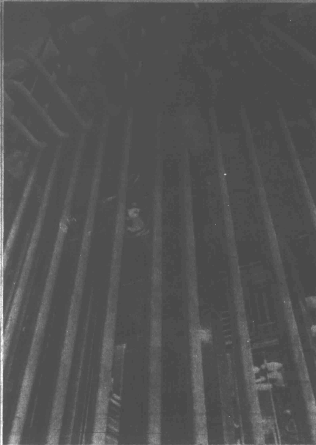
MAZE OF PIPES — A workman emerges behind a maze of pipes in the resin plant at PPG Industries Coatings and Resins Division's new Oak Creek, Wis., complex. The pipes carry resins from processing through final blending to shipping or coatings manufacturing areas. The complex, to be fully operational this summer, has an annual capacity of 50 million pounds of resins and 13 million gallons of coatings. (AP Wirephoto.)
