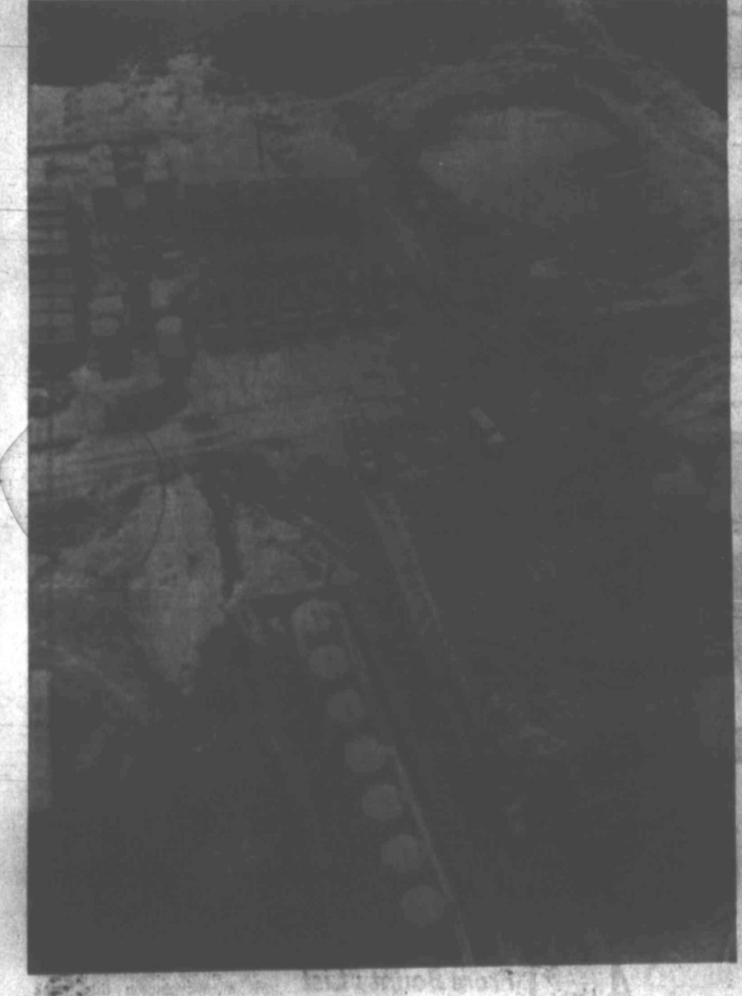
FRACTURING TREATMENT — Aerial view shows a ray of high pressure pumping units being hooked up to pump 900,000 pounds of sand in 500,000 gallons of fluid down a gas well near Marshall, Tex. The massive hydraulic fracturing treatment was performed Tuesday on the Amoco-Jones Gas Unit No. 3 in the Woodlawn field. Massive fracturing techniques have been used by Amoco in the Rockies recently, but Tuesday's stimulation treatment, in the planning for six months, was the first in the Southwest. Spokesmen said tests dictated use of the technique, designed to unlock gas deposits from "tight" formations. (AP Wirephoto.)
