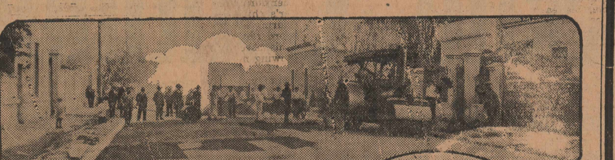
LAYING THE "HOT STUFF" FOR ASPHALT PAVEMENT IN AVELLANEDA, ARGENTINA, SHOWING WAGON OF "HOT STUFF" IN BACKGROUND
