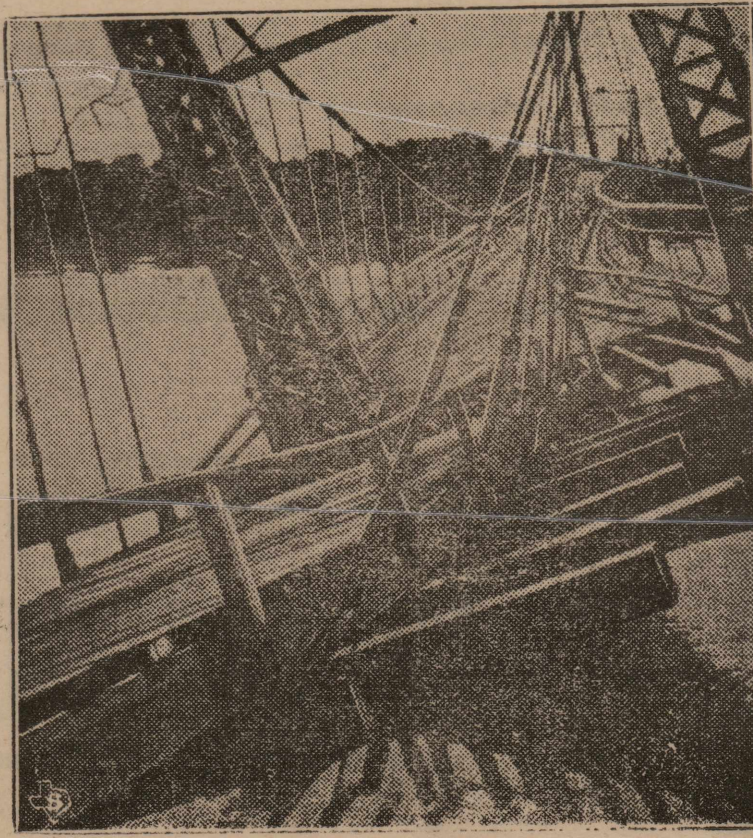
Here is the International bridge across the Rio Grande between Hidalgo and Reynosa, Mexico, pictured after piers on the American end, apparently undermined by recent flood waters, suddenly sank into the mud. No one was on the bridge at the time and no injuries resulted. Repairs are now being made.
