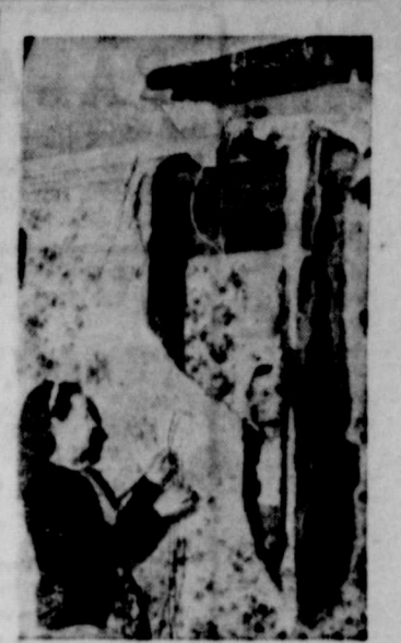
BOLT FROM SKY... Joseph Fey peers through aperture left in George Sunmacker home, South Gate, Calif., by bolt of lightning that traveled down TV antenna. California recently received rain, storm, snow, hail, sleet, thunder and sunshine.
