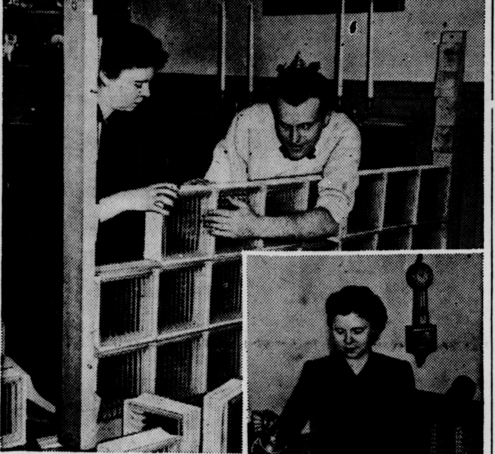
The Brothersens team up to erect a glass block and wood strip partition for the big living room of their apartment.
