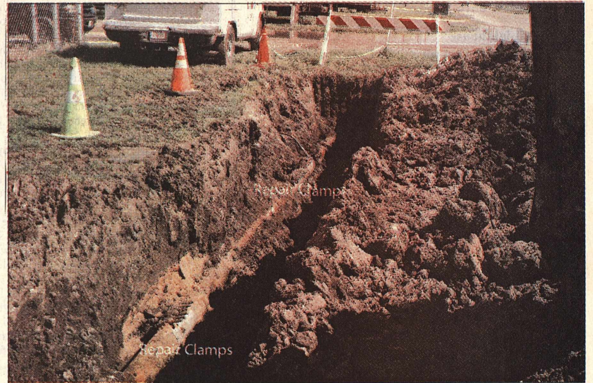
This section of pipe, located near G&L Tool, contains more than 5 clamps to repair the leaks
