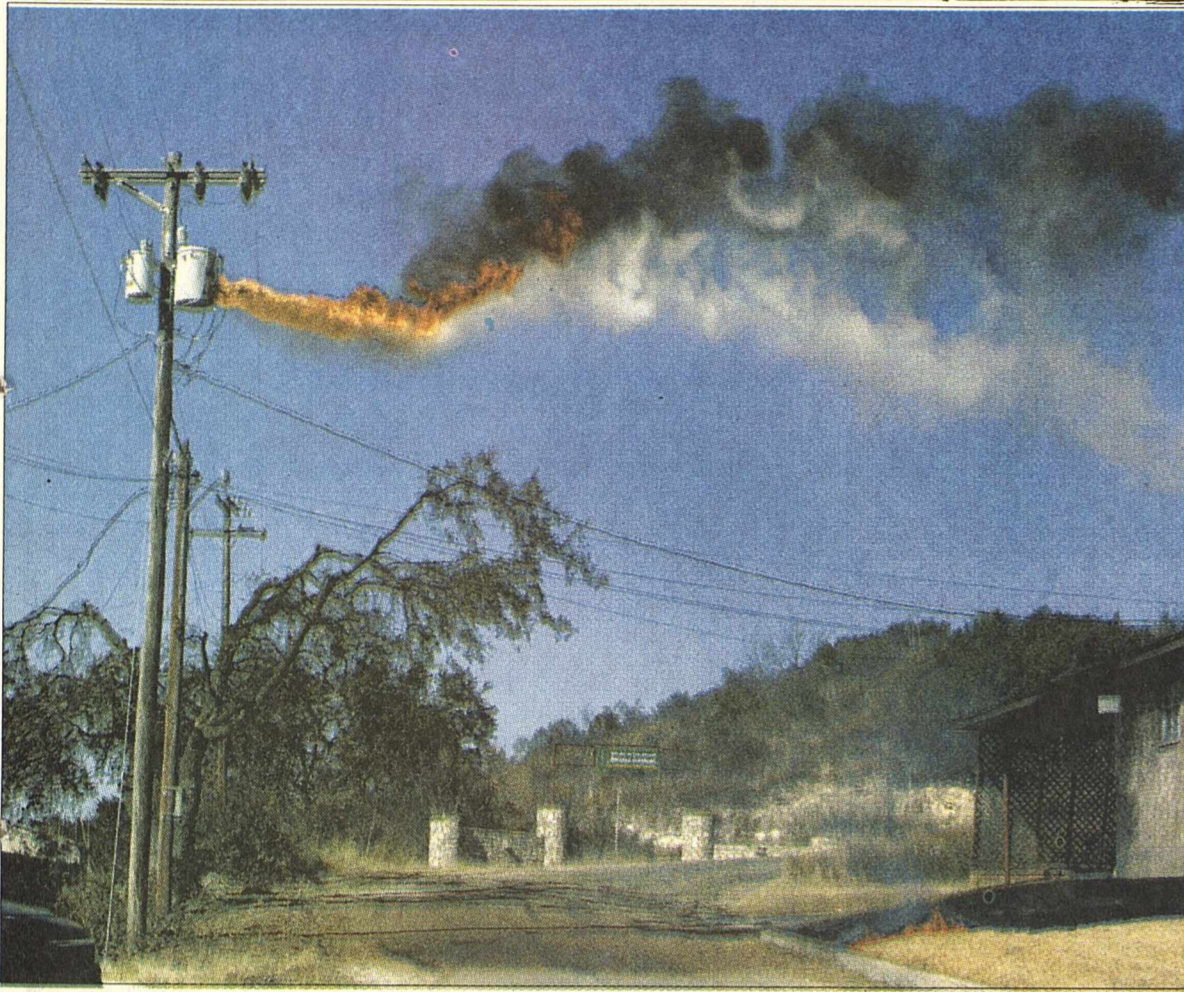
A transformer blows on Mulberry Street, setting a nearby yard on fire. Photo by Storie Sharp
