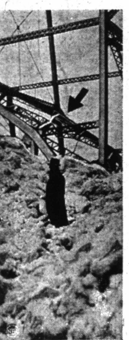
Bulging under the crushing pressure of the mighty ice jam, a score or more steel girders of Niagara's single arch span Falls View Bridge snapped finally. One is indicated by arrow.
