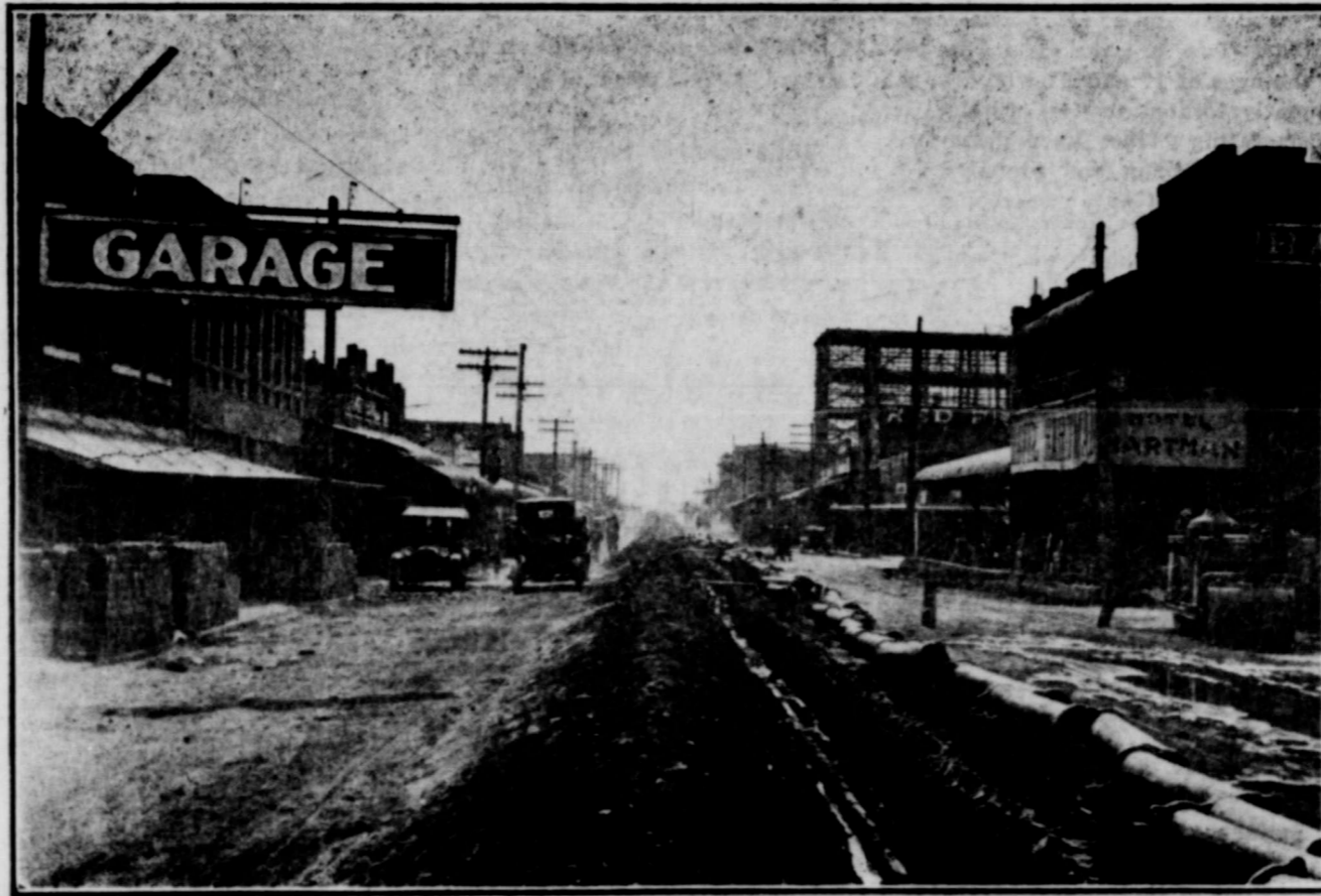
The above picture was made last week showing the old water main in the ditch, and the new pipe lying along side the ditch, which is now being connected. The new five story home of the Cisco Banking Company now under construction can be seen in the back-ground.
