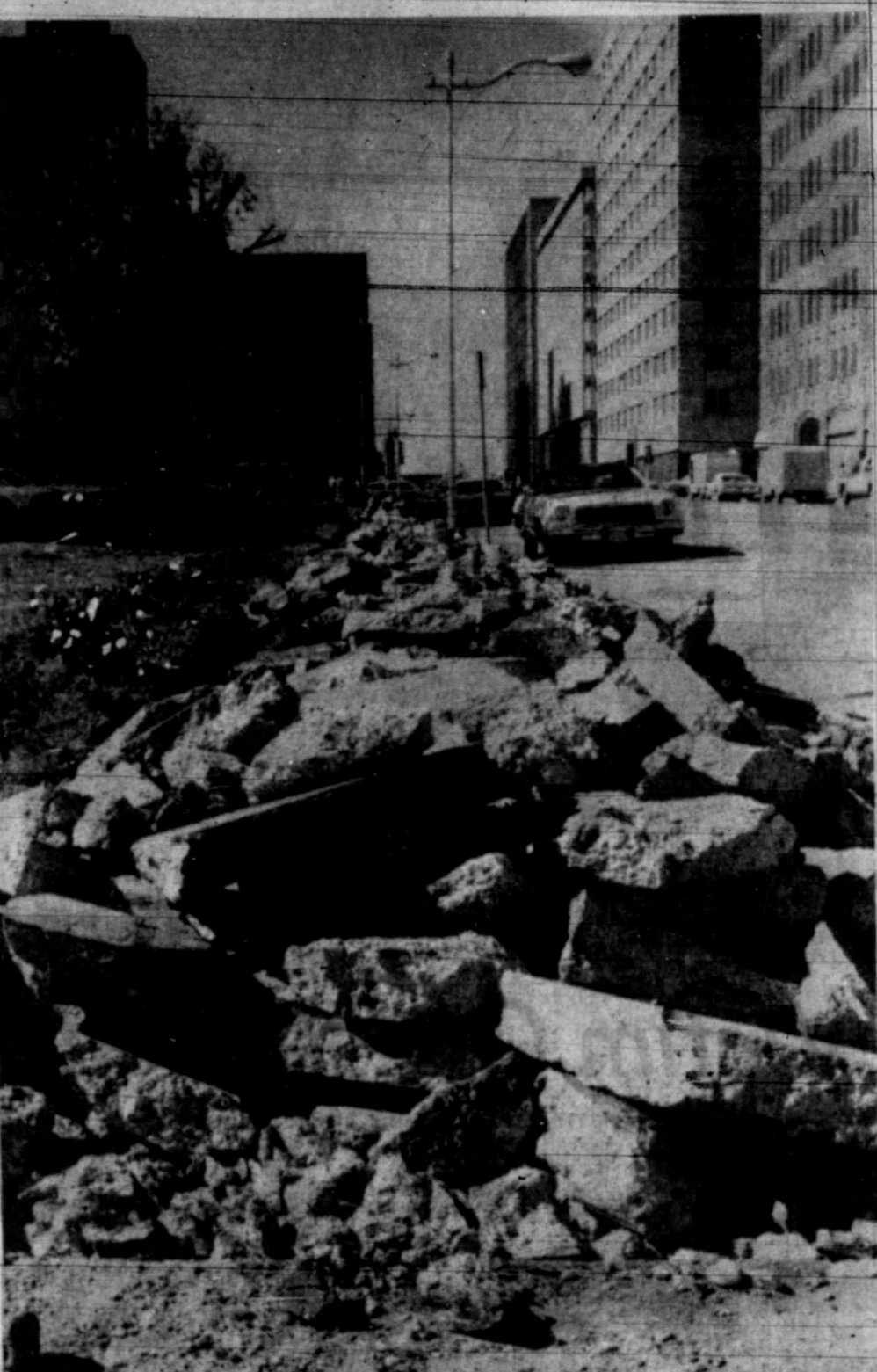
CONCRETE JUMBLE — This used to be the sidewalk on the north side of the Midland County Courthouse, but today it resembles a disaster area. Workmen are tearing out the old walkway and it will be replaced one side at a time over the next four to six weeks, County Commissioner Winfree L. Brown said. (R-T Photo by Charles McCain.)
