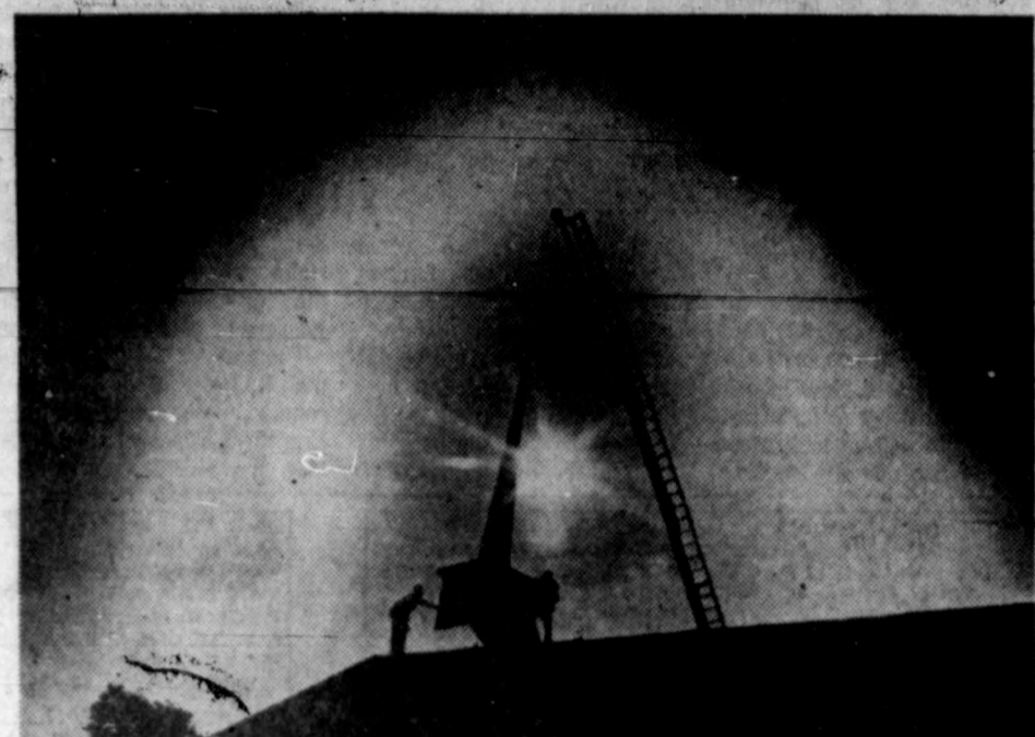
APPROPRIATE HALO — An appropriate halo effect silhouettes a scene atop the roof of the First United Church of Christ in Fremont, Ohio, where workers install a 23-foot steeple during the early morning. (NEA Photomat)
