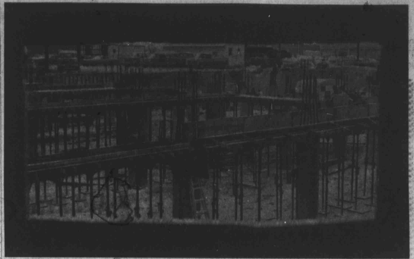
VIEW THROUGH WINDOW — This is what the construction activity looks like at the site of the Midland Hilton Inn, as seen through a window in the sidewalk barricade.
