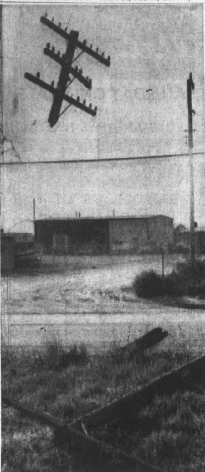
DANGLING POLE — This unusual scene in the 2900 block of Industrial Street resulted when the trailer came unhitched from a truck driven by D. D. Vaughn of Odessa and smashed into the telephone pole. Vaughn was unhurt.
