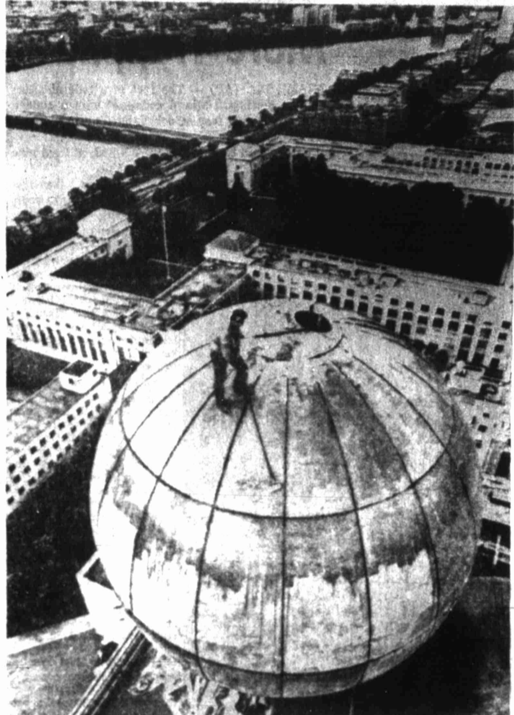
TOP OF THE WORLD—Steeplejack Stanley Stokler of Woonsocket, R.I., goes about the job of painting the dome housing the weather radar atop the 20-story Green Building at Massachusetts Institute of Technology in Cambridge, Mass. The 26-foot dome is made of fiberglass. The Charles River is seen in the background. (AP Wirephoto.)
