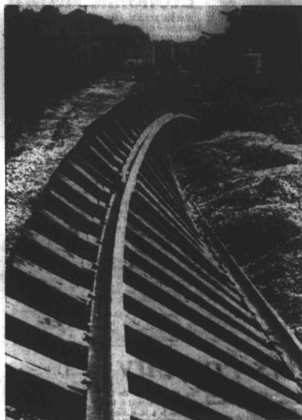
FLOOD RAVAGES TRACK—Extensiveness of flooding of Kickapoo Creek near Peoria, Ill., is shown by a section of washed-out railroad track. This photo was taken shortly after the floods, which caused millions of dollars in damage recently. (AP Wirephoto.)
