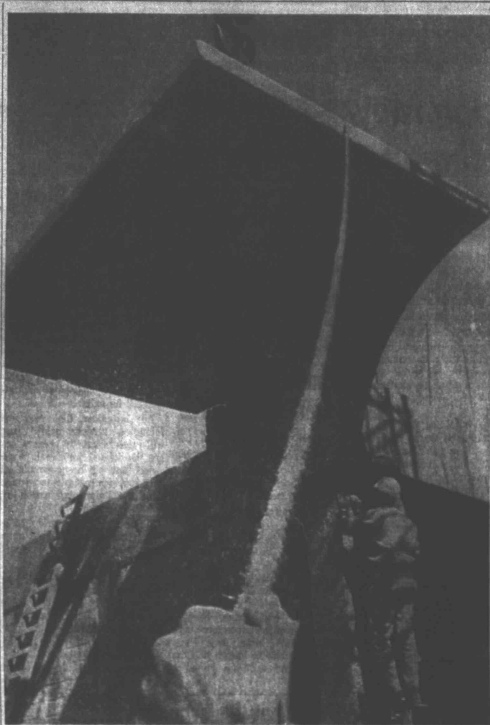
CONCRETE KITE — What may appear to be a giant kite is actually a 32,000-pound precast concrete section of the entrance portico covering being fitted at the Permian Basin Petroleum Museum, Library and Hall of Fame under construction south of Midland. The job of casting is said to be a "first" due to the curve and weight of the sections.
