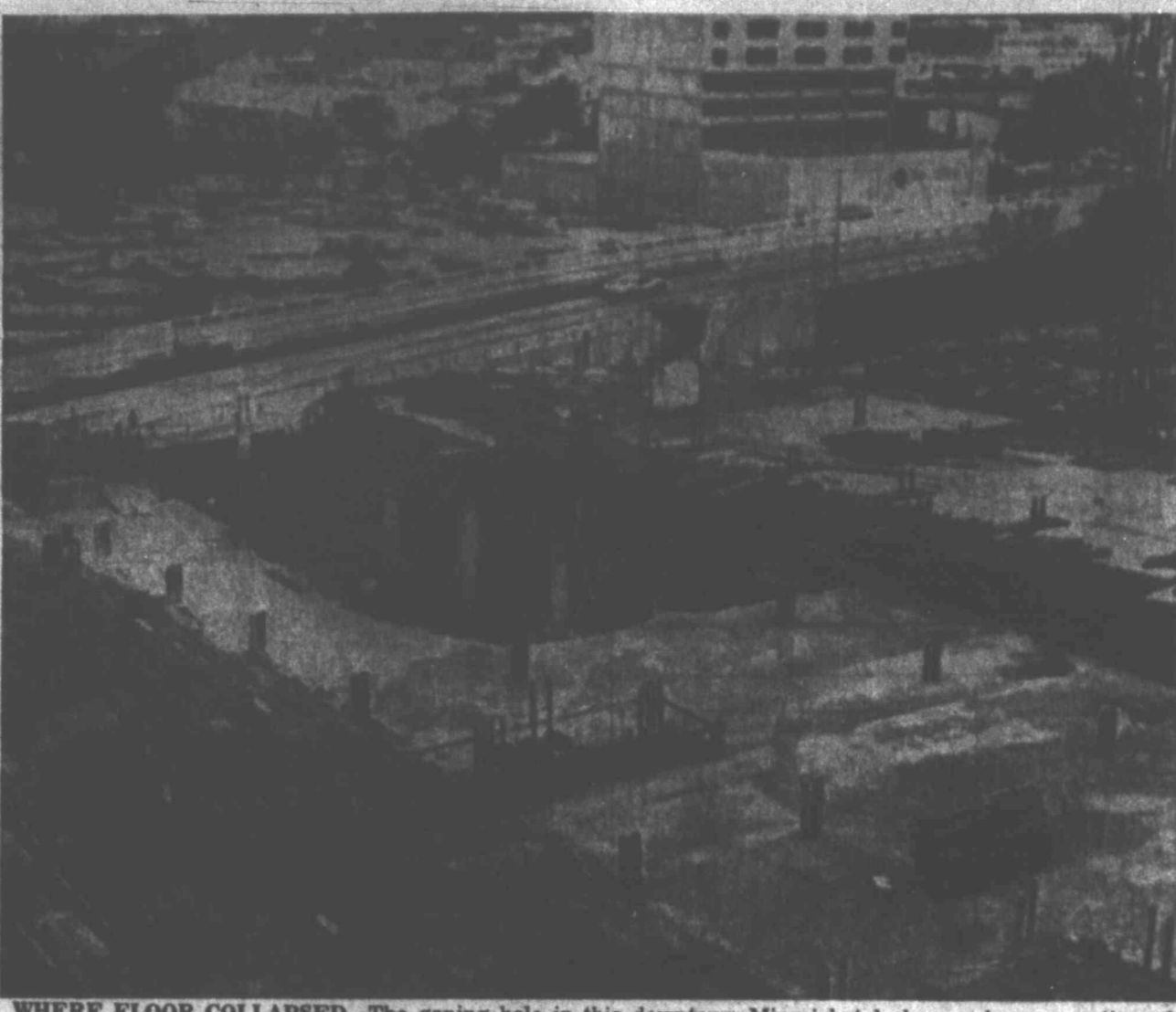
WHERE FLOOR COLLAPSED—The gaping hole in this downtown Miami hotel shows where a section of the second level collapsed Monday afternoon as concrete was being poured. Miami police said seven workmen were injured. (AP Wirephoto.)
