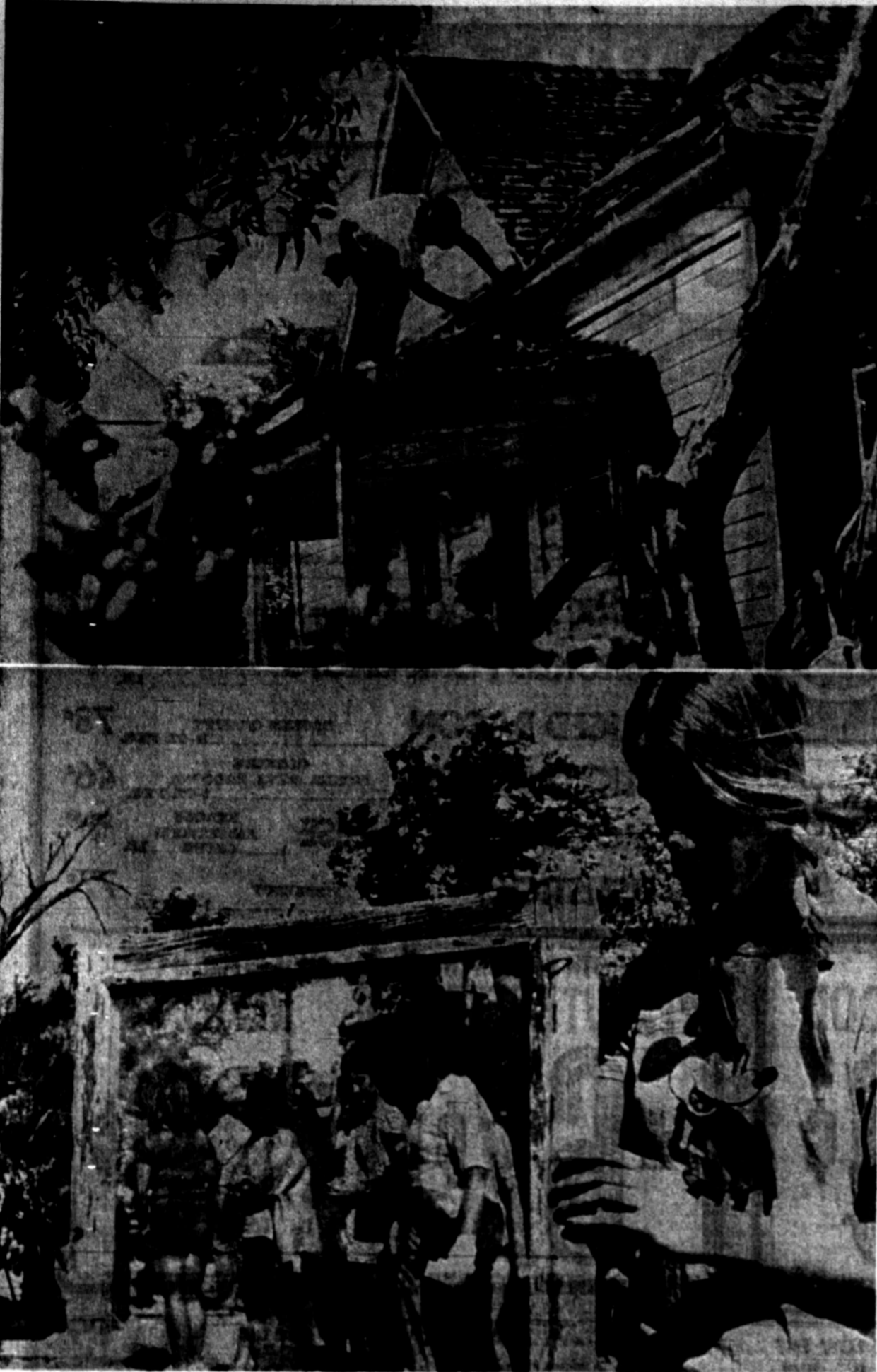
CHRISTMAS IN APRIL — Scores of volunteers from churches, businesses and civic groups repaired 25 homes of elderly Midlanders Saturday during the "Christmas in April" project. In top photo, a worker repairs a roof. In bottom photo Jacque Thams works on a window screen. Youths and adults alike worked on the followup to last year's "Christmas in October."
