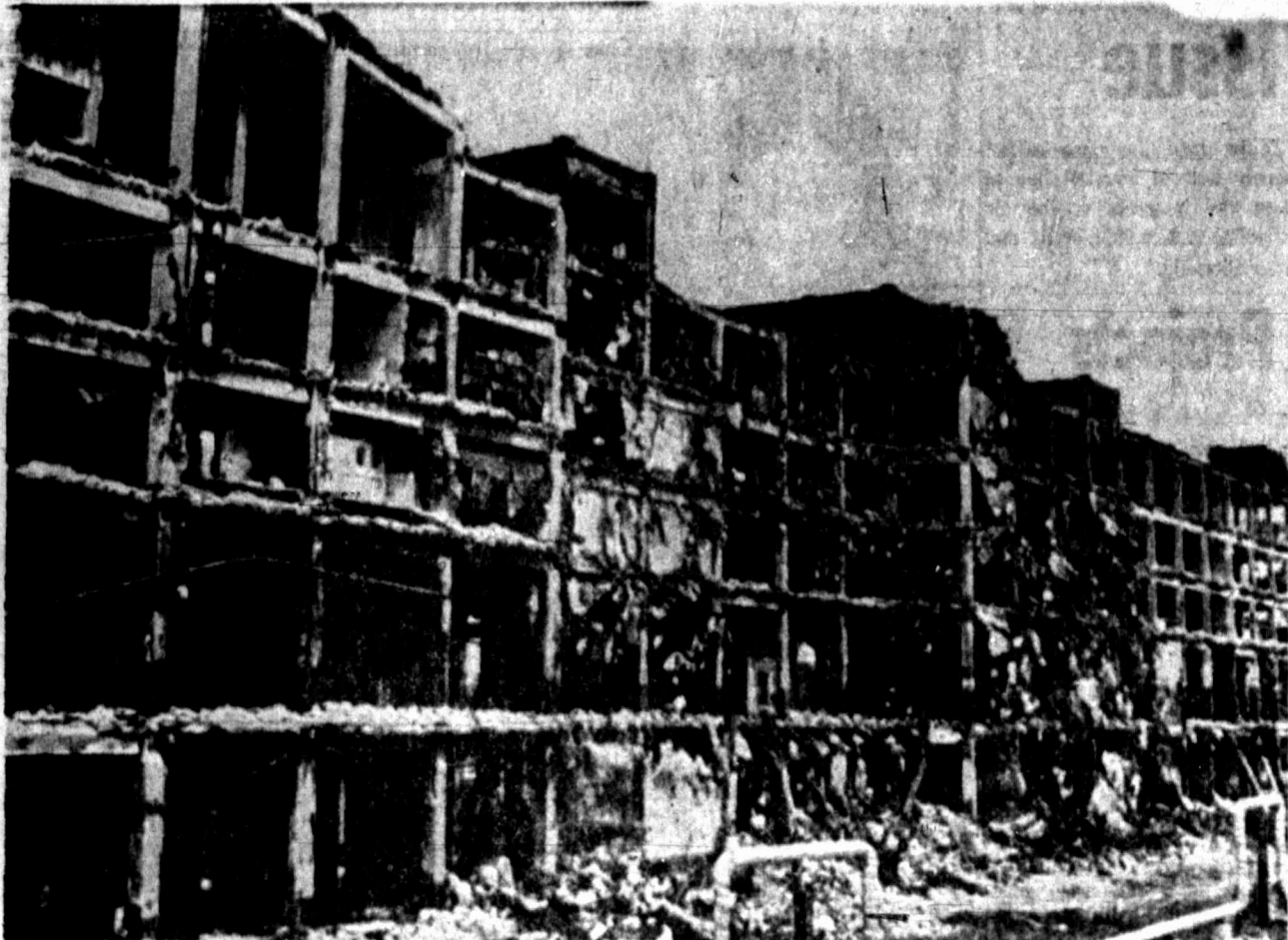
DEMOLITION ON A GRAND SCALE — The old Burlington Railroad freight house in Chicago, which has been unused for some time, presents this pattern of squares as it is being razed. The structure occupied a full block along the Burlington tracks south of the Chicago's downtown district. (AP Wirephoto.)
