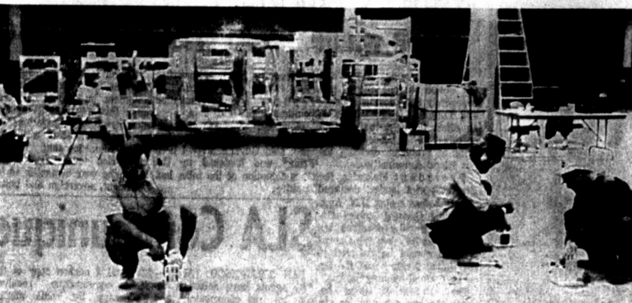
GETTING READY FOR MOVE—Workmen install outlet equipment for automatic mailing machines to be installed in the new United States Post Office nearing completion here. From left are Mike Burns and Dave Clark of Big Spring, and J. L. Samples of Midland. Postmaster David Holster said the move to the new building will begin April 24.
