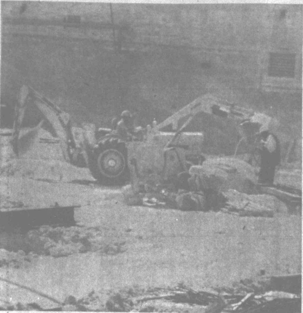
WORK PROGRESSING — Workmen are busy in what will be the basement area of Southwestern Bell Telephone Co.'s multi-million dollar seven-floor building which will be used for expanded telephone facilities in the Tall City. The project is under way at Missouri and Big Spring streets. Completion of the building is still many months away.
