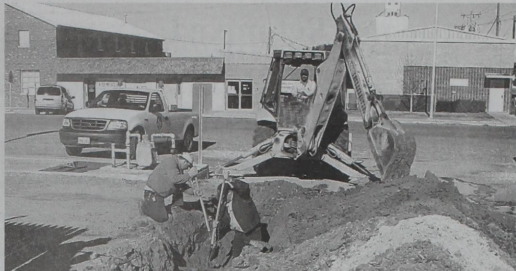
City employees dig a ditch for a new sewer line going to the Bailey County Courthouse recently.
