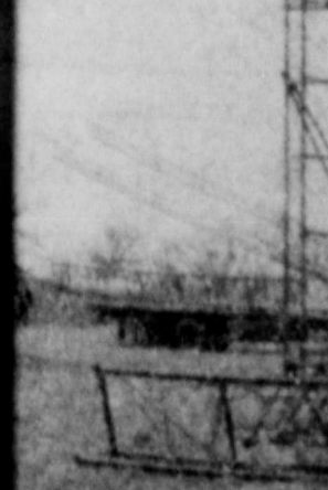
UP—Pictured here is the 300-foot tower being constructed by Telco, which will provide
