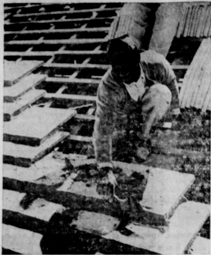
BUILDING A BERMUDA ROOF — A workman cements into place one of the finely-cut slices of Bermuda limestone which compose Bermuda's distinctive roofs. When completed the roof will be whitewashed and fitted with a drain which will funnel rain-water into a storage tank, providing the owner with his supply of fresh water. All Bermuda houses are required, by law, to have a sloping white roof to catch drinking water. This gives the Bermuda landscape a quaint, harmonious charm almost unique. F.N.S.
