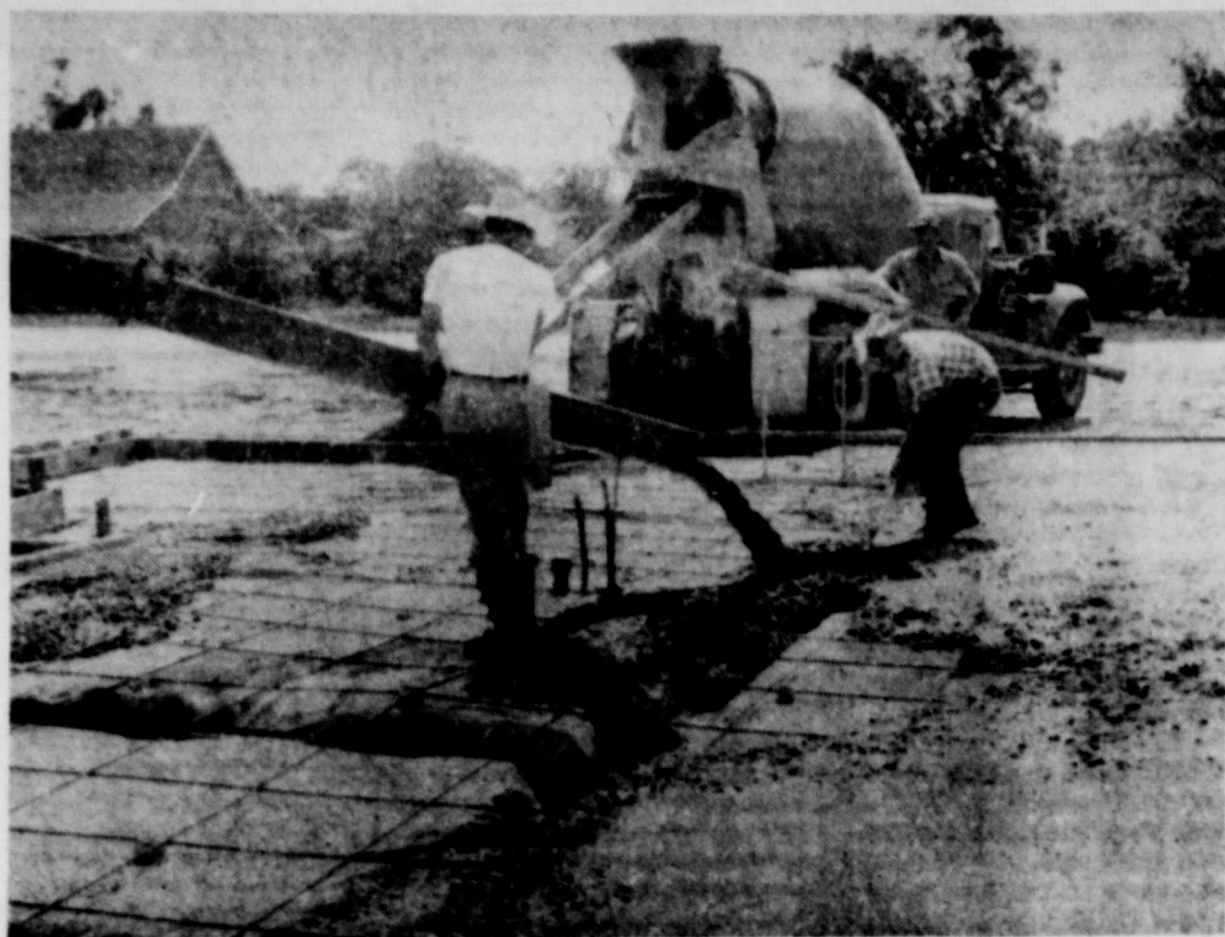
GOING UP—Shown here are workmen as they poured the last of the concrete for the foundation of Hico's new post office
