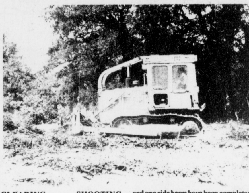
CLEARING SHOOTING RANGE —David Nichols of Nichols Dozers works at clearing the location for the rifle range at the Callahan County Shooting Range between Clyde and Baird on FM 18. To date, the backstop
