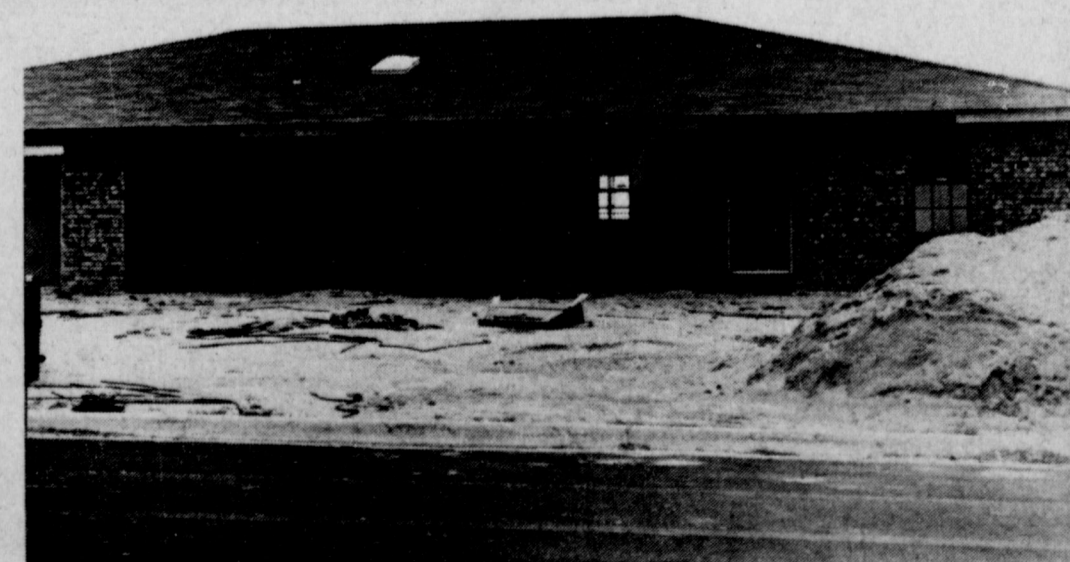
SPS HOME CONSTRUCTION---Several of the engineers with the construction of the Southwestern Public Service Company's new coal fired generating plant near Muleshoe are construction in the new Parkridge Addition. This home is nearing completion at this time, and the other homes are in stages from foundations to framework going up.
